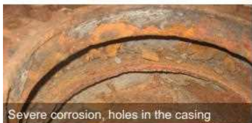
Main circulating water pump
