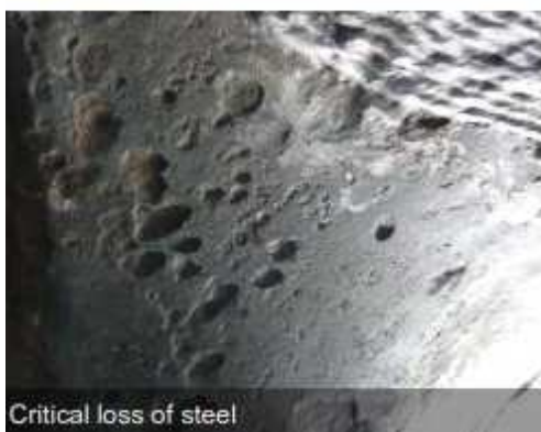
Severe corrosion of exhaust pipe
