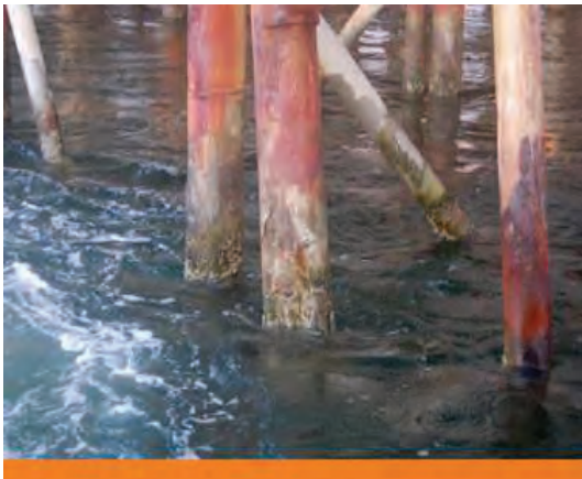
Splash Zones Common Problems Risers and platform legs are subject to severe damage...
