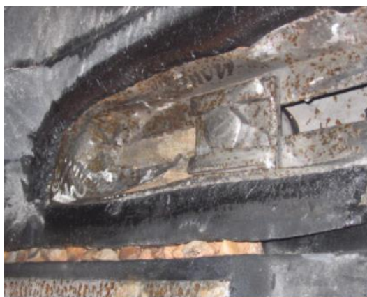
Damages to grinding mill lining
