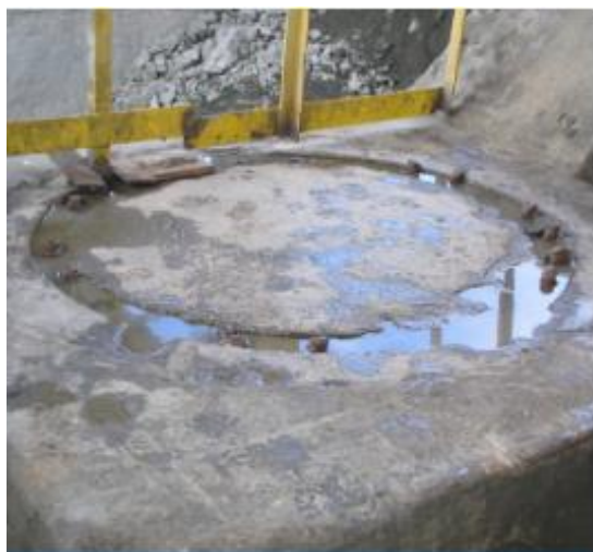
Damaged concrete base
