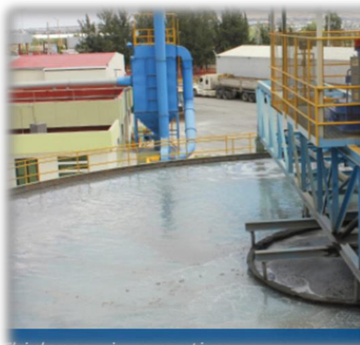
Thickeners in operation
