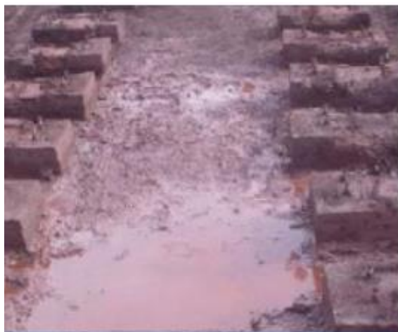
Damaged bases of railroad tracks
