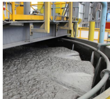
Equipment under chemical attack
