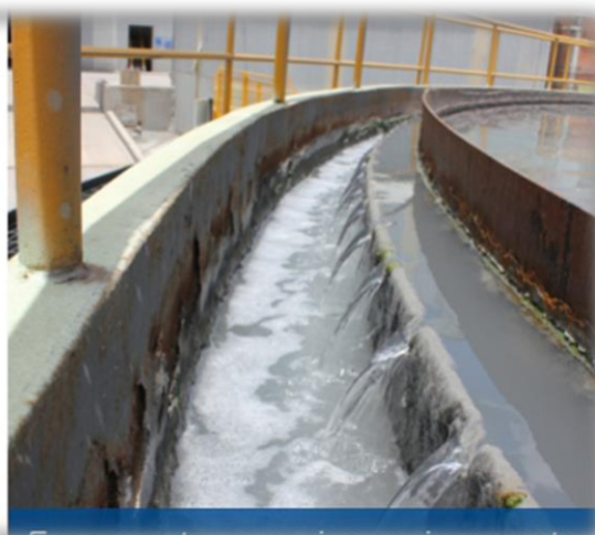
Exposure to corrosive environments
